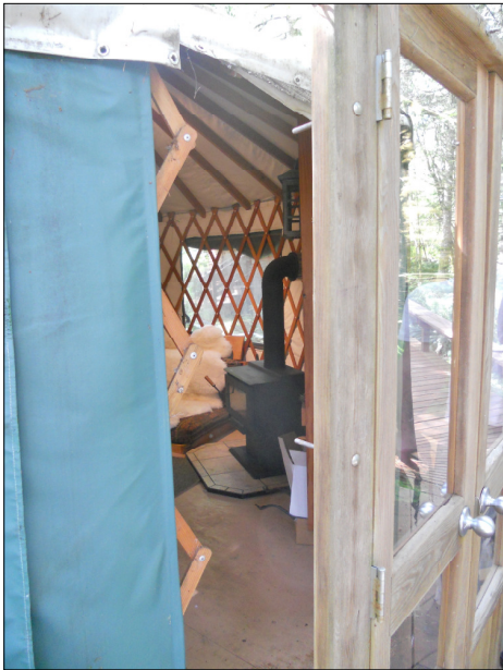
2. Entire door frame pulls out of the yurt.
